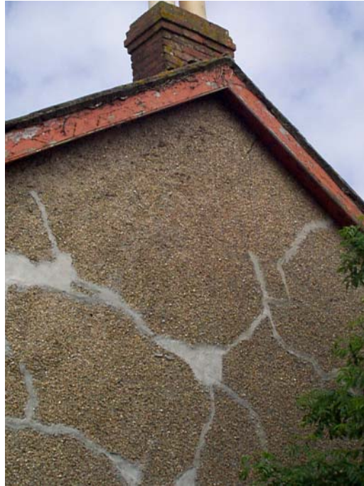
Figure 2-14. Irregular branching cracks (many recently repaired) in render overlying seriously degraded blockwork. The aggregate is a sulphide-rich copper-arsenic mining waste typical of the northern part of the Camborne - Redruth mineralised district. House near Camborne.
