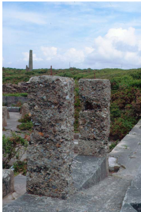
Figure 2-18. Mass concrete pillars in ruined mill buildings at West Wheal Kitty Mine, near St Agnes.
