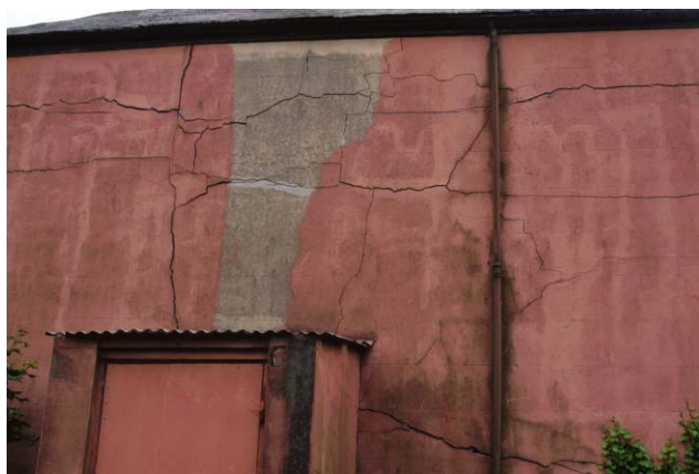
Figure 2-15. Wide branching cracks in render overlying severely degraded mass concrete. The aggregate is a very coarse, low fines copper mining waste. Commercial property in Camborne.
