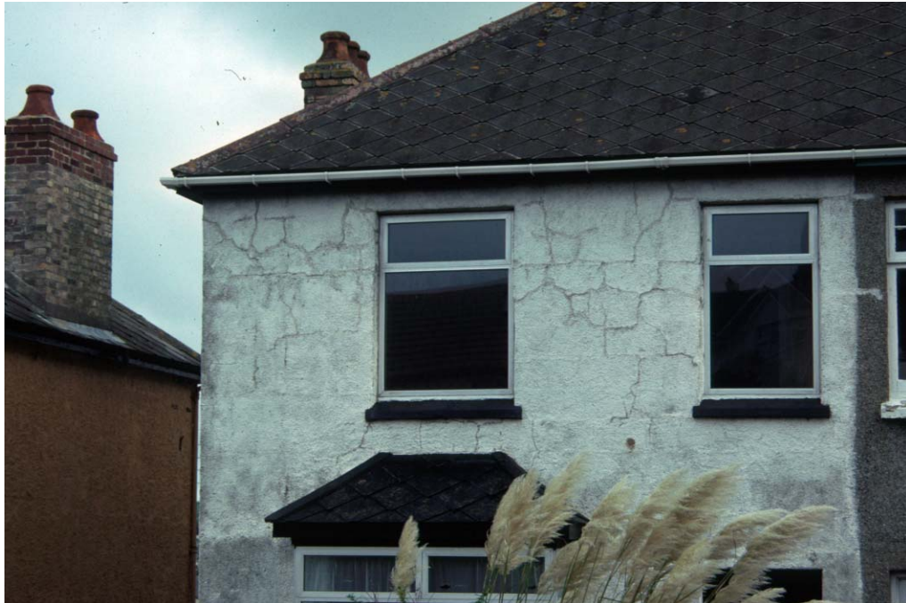
Figure 2-16. Severe cracking in render overlying blockwork. The cracks commonly follow mortar joints between blocks in the underlying wall. This type of render cracking is characteristic of degradation of blockwork made with lead ore processing wastes in the Perranporth area and East Cornwall. House at Perranporth (now demolished).
